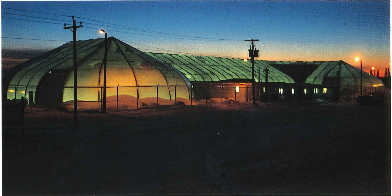
For a year-long project to destroy PCBs in soils and materials, OHM shipped its mobile infrared incinerator, laboratory, and support equipment by barge 1,600 nautical miles to Goose Bay, Labrador, where the company designed and built this 40,000 square foot facility.
