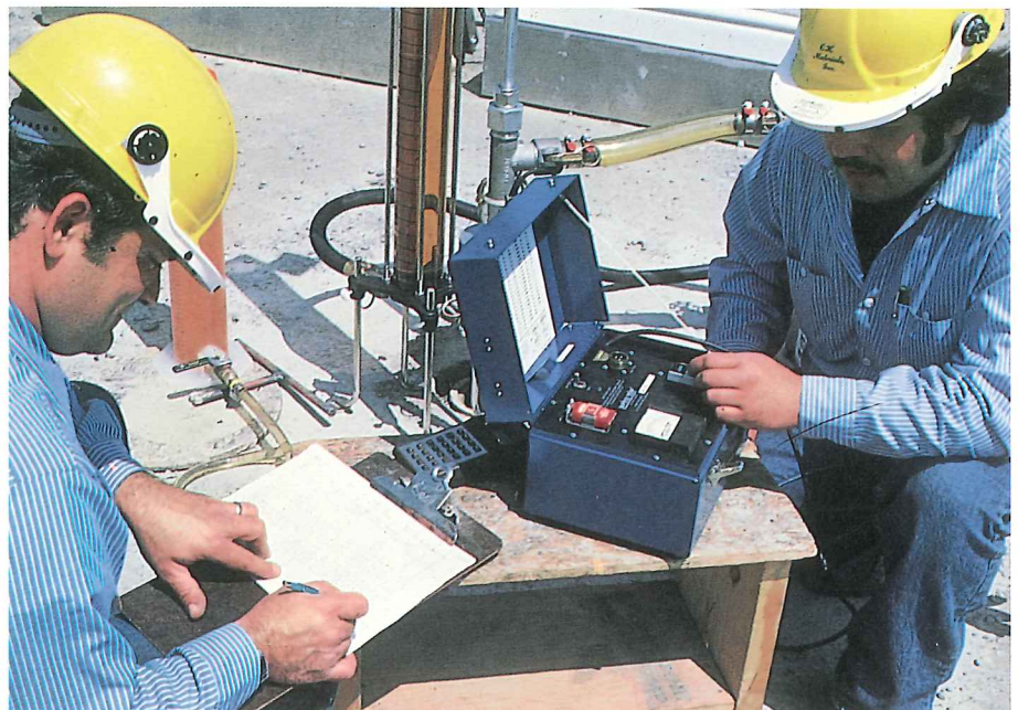
Certified OHM technicians use the proven PETRO TITE ® system to perform precision leak testing of underground tanks.
