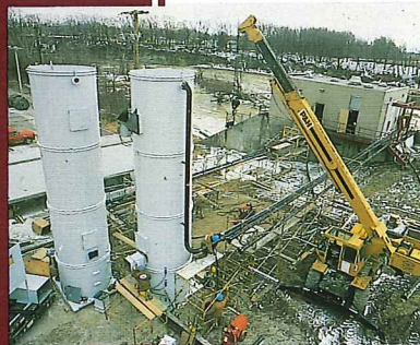
Design, fabrication and operation of 5 million-gallon-per-day water treatment system for toluene released by pipeline leak.
