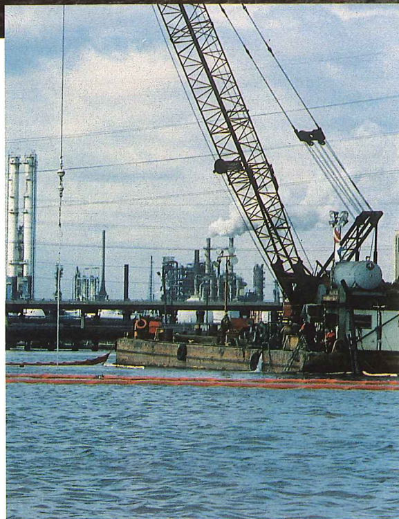
Major waterway spill cleanup of 500,000 gallon diesel fuel spill from underwater pipeline release.
