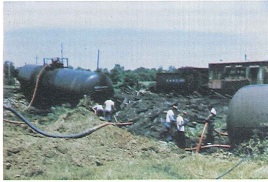
Transfer and spill cleanup of nearly 50,000 gallons of a variety of oil products were accomplished despite the remoteness of this derailment.
