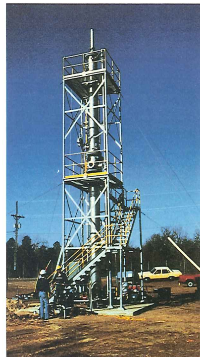
Custom designed air stripping tower removing TCE and other volatile organics from groundwater
