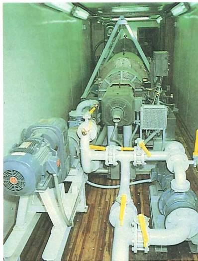
Mobile equipment for sludge dewatering
