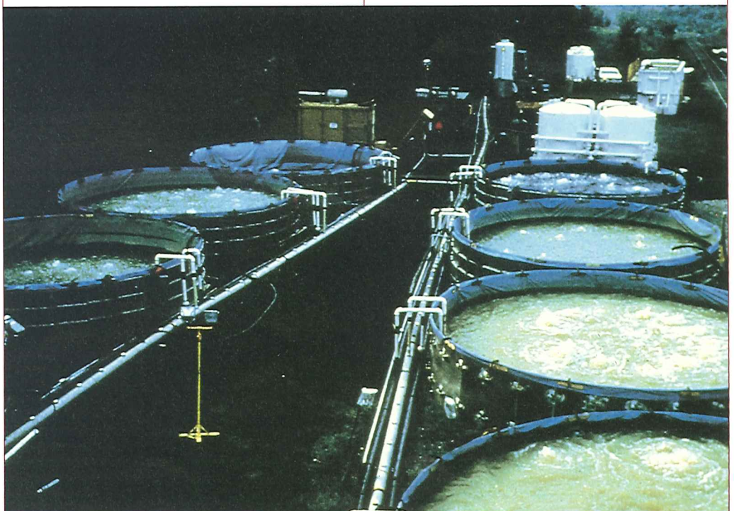
Mobile treatment systems used to detoxify groundwater
