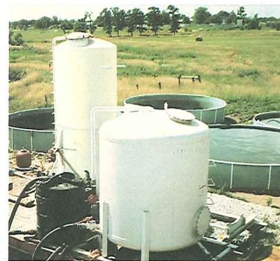
Biological treatment tower and associated treatment equipment.
