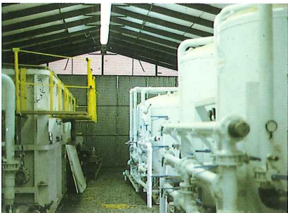
On-site treatment systems can be housed in portable buildings for year-round operation.
