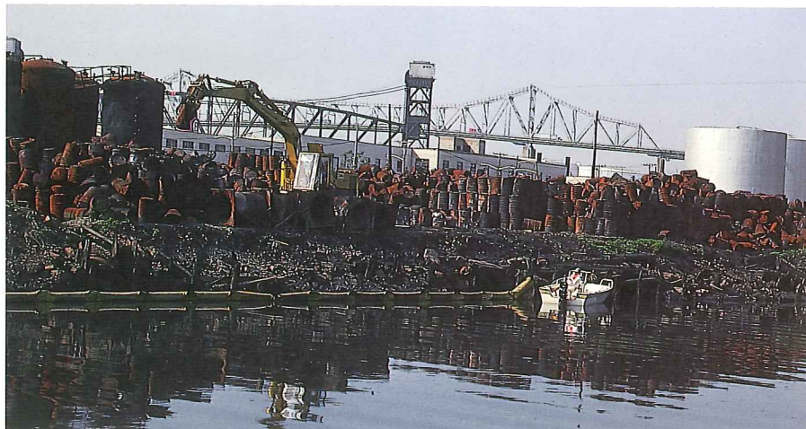
OHM enhances project safety and productivity by the use of mechanized material handling systems.
