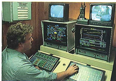
Fully automated, computerized controls and specially trained operator ensure high incineration productivity and regulatory compliance.
