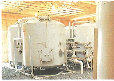
Thirty-million-gallon PCB wastewater treatment project at the Avtex Fibers Superfund site in Front Royal, Virginia.
