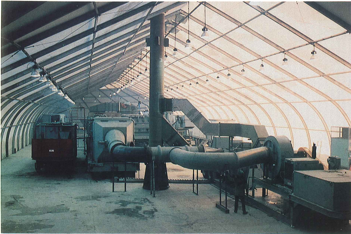
Mobile incinerator that destroyed PCBs in 4,000 tons of soil, transformer components, wood, and drums at DND project. Project took place in 40,000 square foot facility, designed and constructed by OHM.
