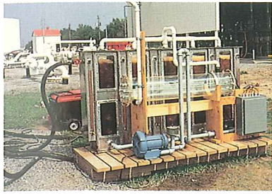
Developmental tank-bottom totally enclosed water treatment system (airlift stripping/ultraviolet destruction) to reduce benzene to below the TCLP standard of 0.5 ppm at petroleum product terminals.
