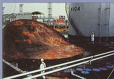
(Above series) Kaohsiung, Taiwan, where OHM removed tetraethyl lead sludge from a 260,000 gallon storage tank, used high-pressure water blasting to remove residue, and dismantled the vessel for disposal.
