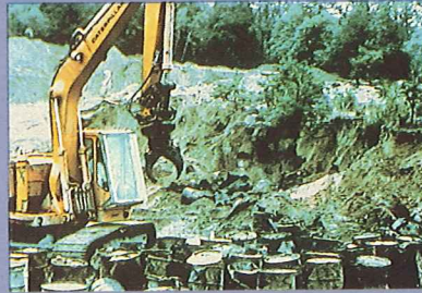
Buried drum removal at the Picillo Superfund site in Coventry, Rhode Island, where OHM subsequently applied landfarming to biodegrade phenolics.
