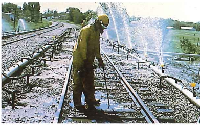
OHM's patented Underground Recovery and Treatment System in operation following a transportation incident
