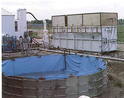
Customized mobile treatment system—clarifier, retention pool and air stripper—addressing solvents leaking from an underground tank
