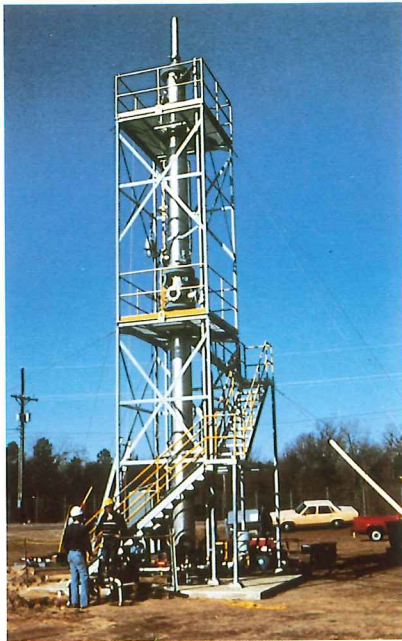
Custom designed air stripping tower removing TCE and other volatile organics from ground water
