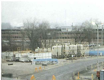
OHM treatment system prior to enclosure for winter operations on a major decontamination project.
