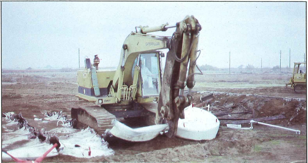
Hydraulic shears are cost effective tools for cutting up tanks, process lines and other structures during decontamination projects.
