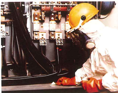
Sampling prior to decontamination of electrical substation equipment involving PCBs.
