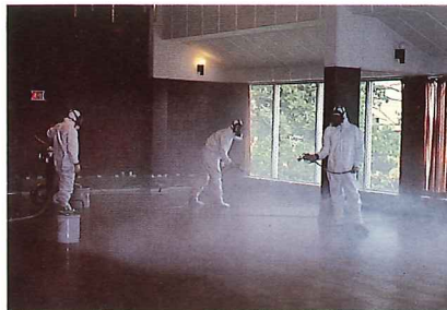
Porous materials after initial surface cleaning can be sealed with an airless application of special sealants.
