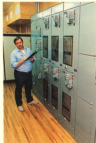
Electrical control system for bioreactors
