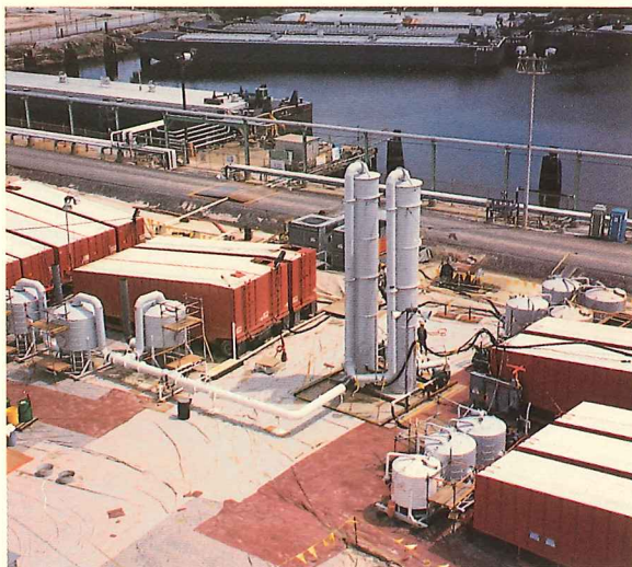
26 million gallon water treatment system designed to meet Louisiana Department of Environmental quality standards
