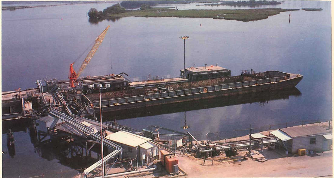
Customized dredge to excavate 18,000 tons of solvent-contaminated river sediments from Louisiana ship channel
