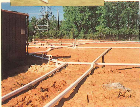
Patented soil vapor extraction system technology for a year-long project in South Carolina selected for cost-effective benefits
